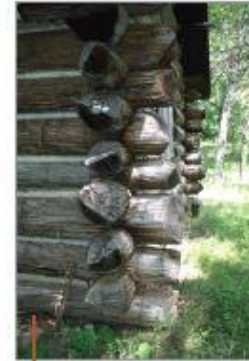
Log construction of the corner of the Carriage House. Zigzag wires were wrapped around the ends of the logs to minimize peeling of the wood and bark.
